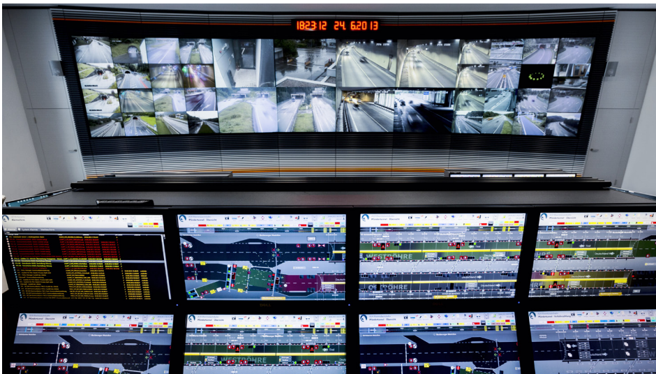
Figure 2: In the tunnel control center, all data and information for monitoring the Pfänder tunnel are consolidated.
